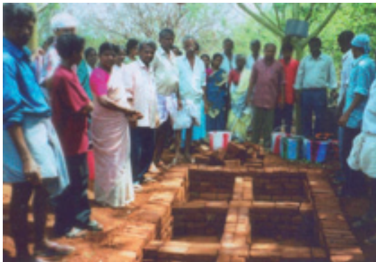
Cow Pat Pit showing brick construction – note the bottom of pit is bare earth.
